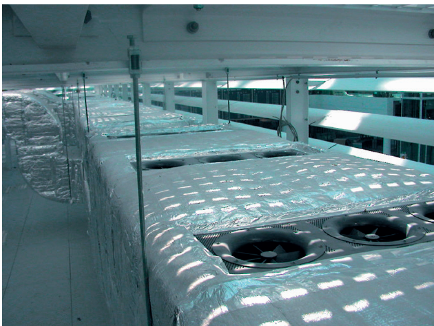
Installation of multi-swirl diffusers in the top side of the supply duct.
